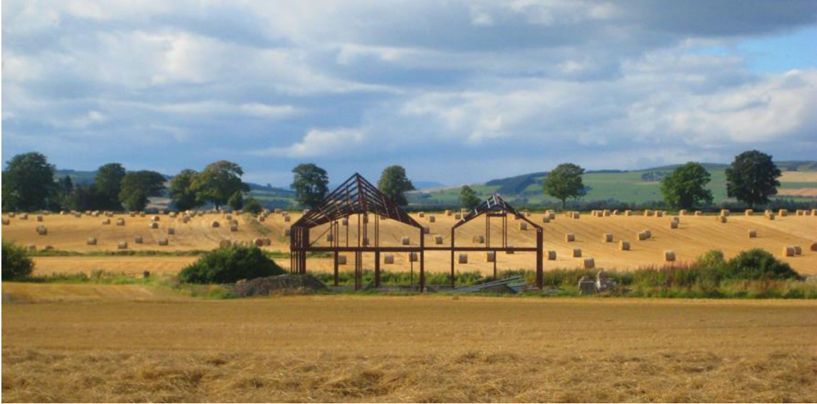
Image 8. Extending local agricultural contractor's skill base, through a principle of 'poetic pragmatism' with regard to structure and construction, was a further fundamental objective of this work. 'The Shed's' parabolic roof is achieved using simple (albeit manipulated) steel frame 'barn' construction.
